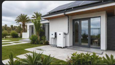
Rooftop PV + storage
